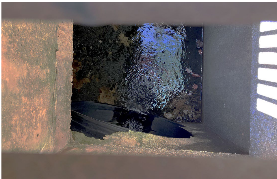
Pipe connecting inside inlet.
