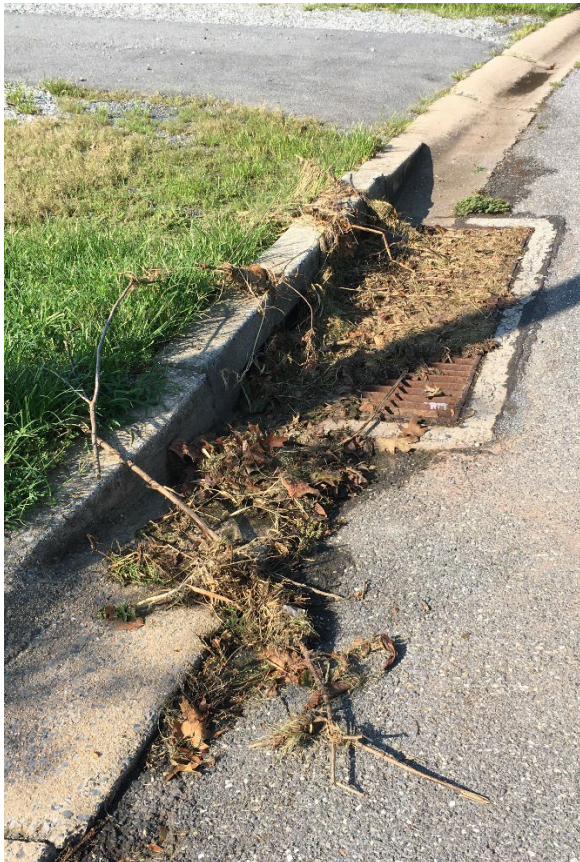
Yard waste accumulating on and around inlet.
