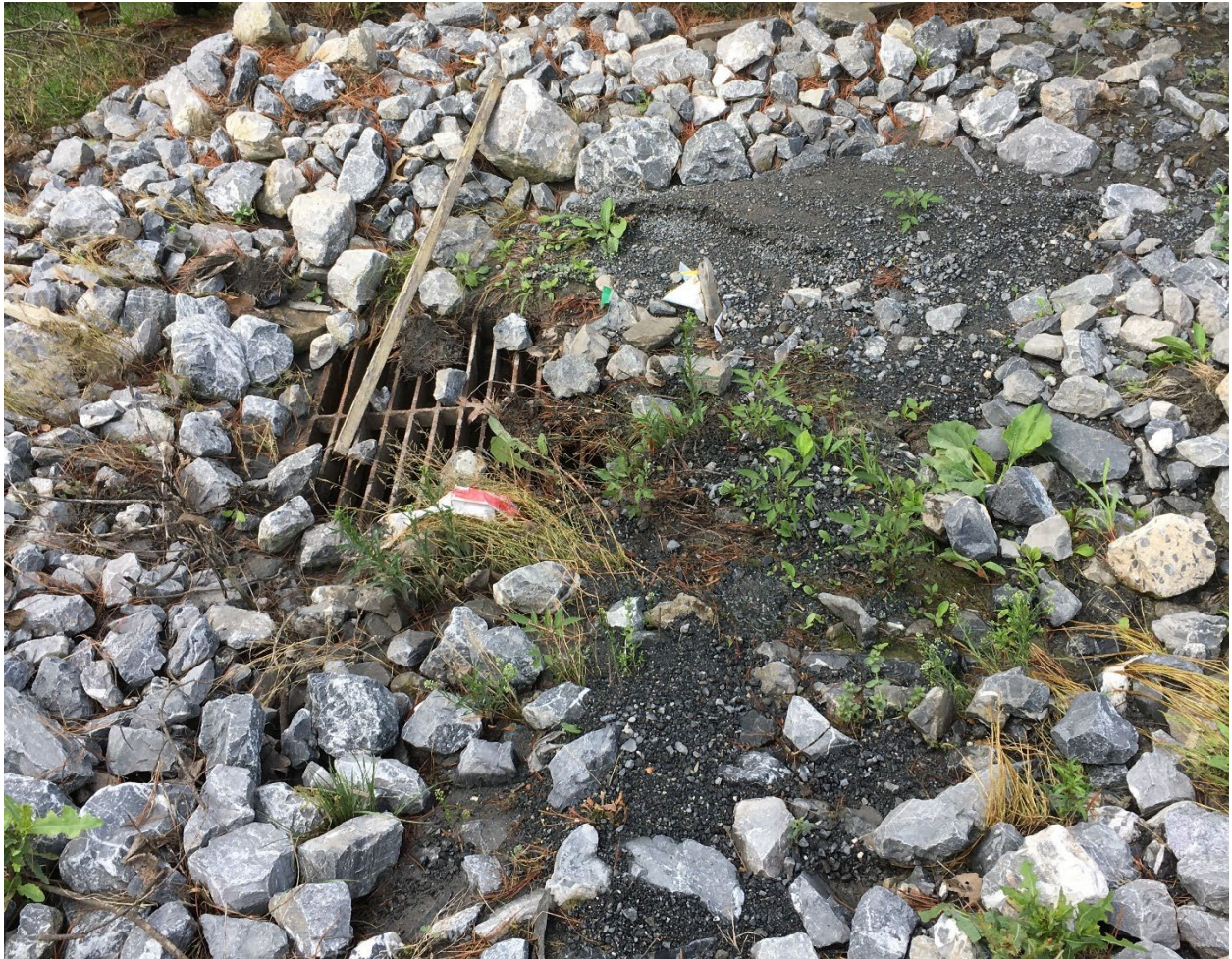
Inlet in landscaping bed nearly covered with stone and other debris.
