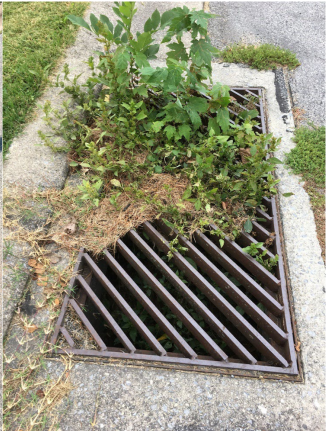
Yard waste on an inlet with long term lack of maintenance, and plants growing through the inlet.
