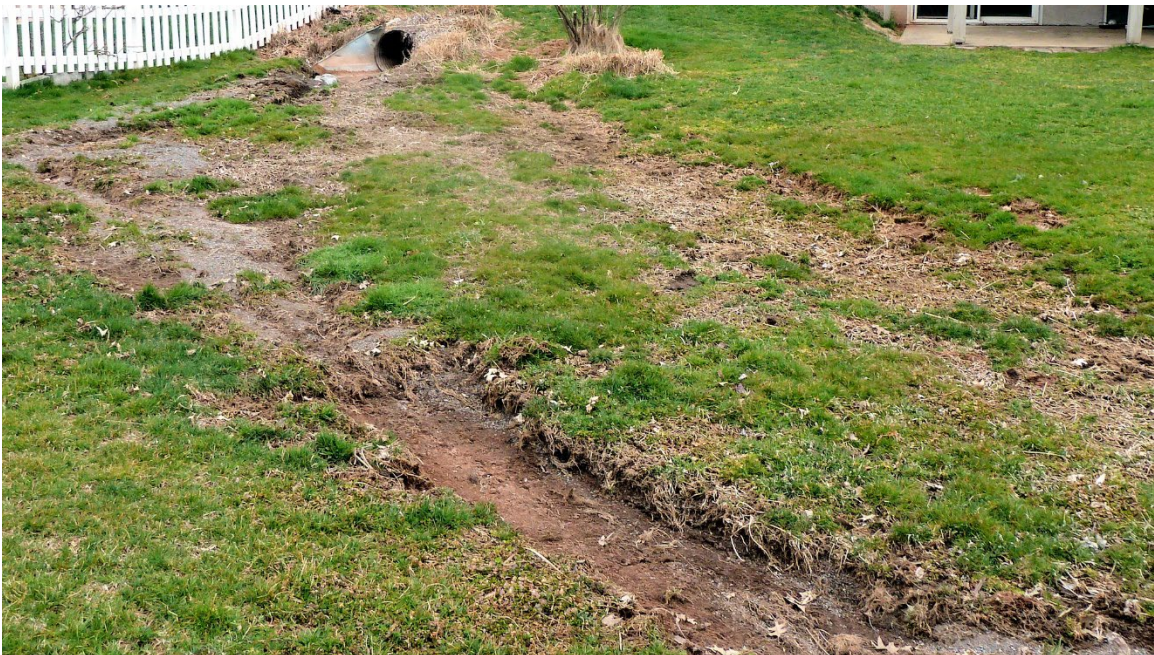
Erosion caused by flow from an inlet into a basin. In this case, the flow rate was too high for the lawn. To repair this so that the problem doesn't return will probably require the installation of protective matting prior to reseeding, or the addition of a rock apron energy dissipator.
